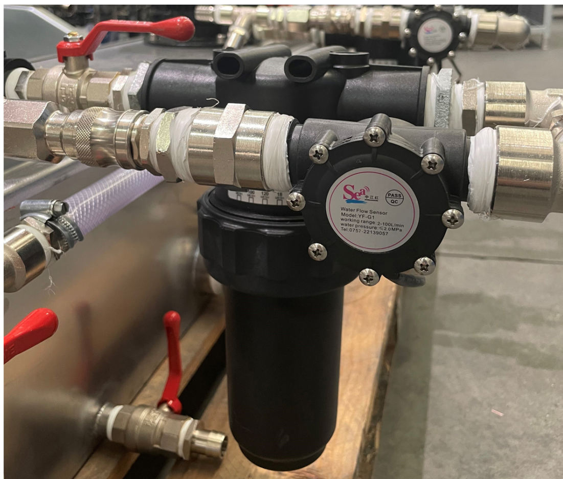
Flow switches to check the filter cleaning status
